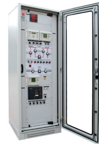
SWS - Interior Cabinets for HV substations
